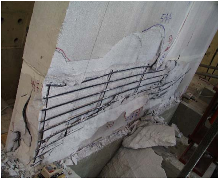
Figure 5.71: Buckling of welded-wire reinforcement in Shear Wall Specimen 9
