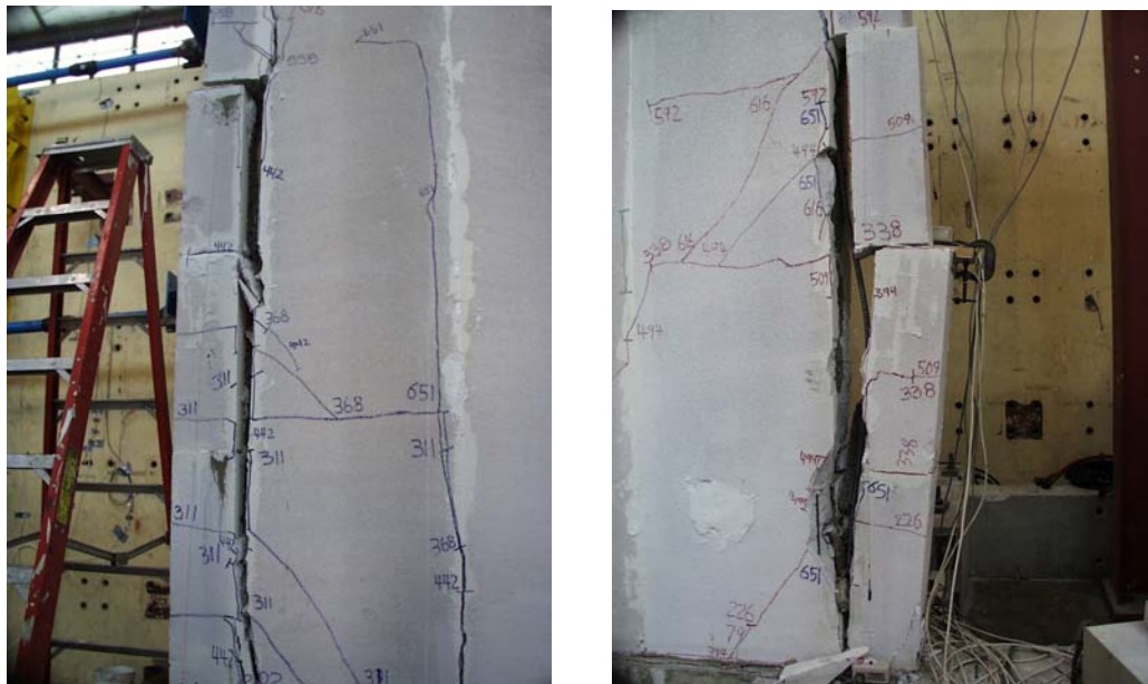
Figure 6.35: Loss of modular block columns on the north and south ends of Shear Wall Specimen 15b
