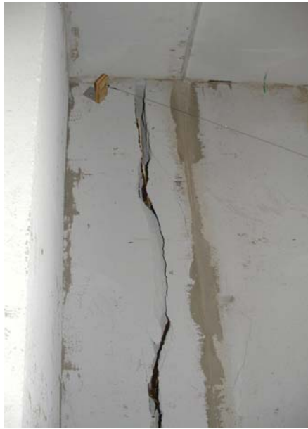
Figure 8.9: Vertical crack at north end of east wall (top of first story wall)
