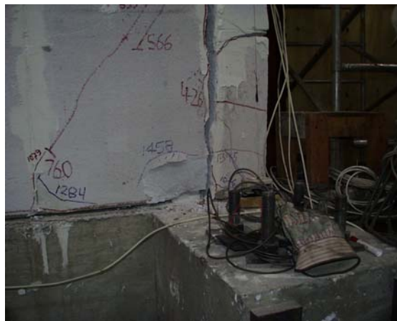
Figure 7.35: Loss of end block on compression toe in Shear Wall Specimen 16
