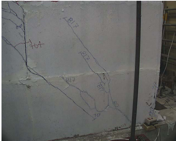
Figure 5.41: Gap in head joint of second course indicating sliding in Shear Wall Specimen 4
