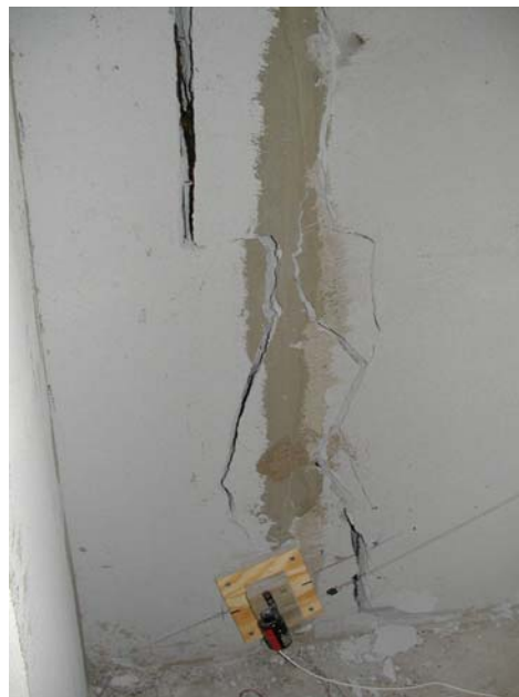
Figure 8.10: Vertical crack at north end of east wall (base of first story wall)
