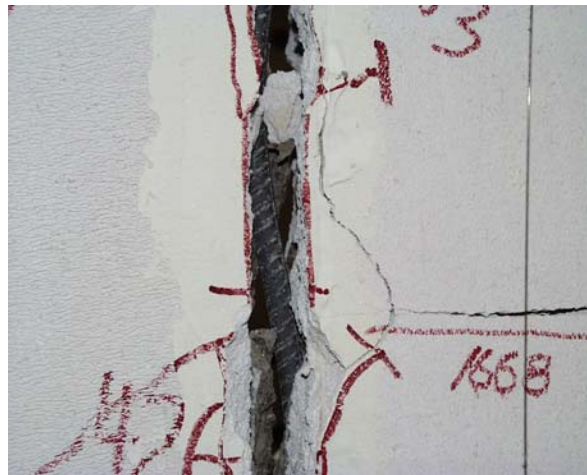
Figure 6.44: Buckled reinforcement in Shear Wall Specimen 16
