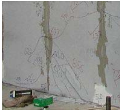
Figure 8.8: Example of diagonal cracks and spalling at dowel location
