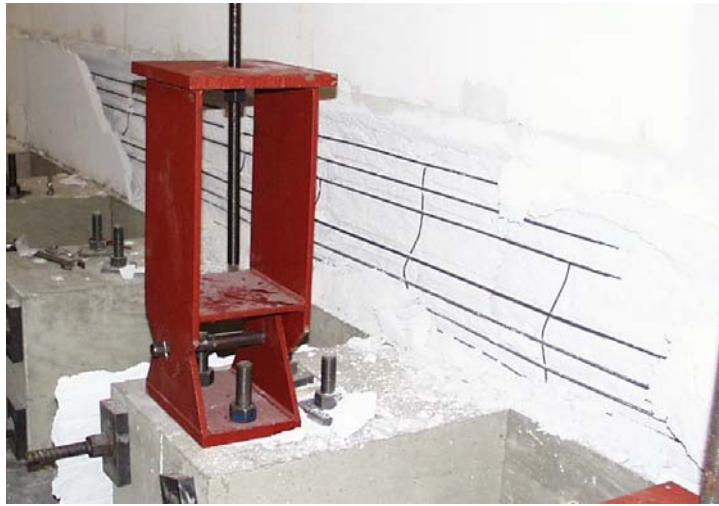
Figure 5.10: Buckling of vertical welded wire reinforcement in Shear Wall Specimen 1
