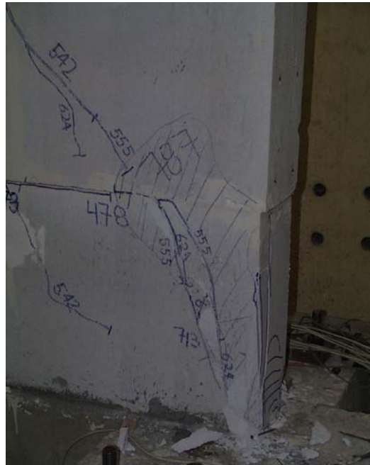
Figure 6.14: Crushing of the compression toe in Shear Wall Specimen 14a
