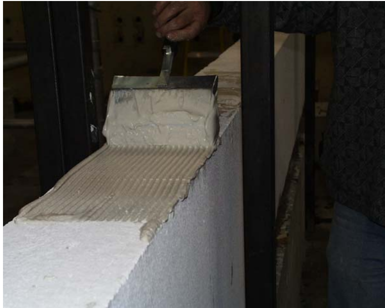
Figure 2.7 Placing a layer of thin-bed mortar on AAC panel in Shear Wall Specimen 1
